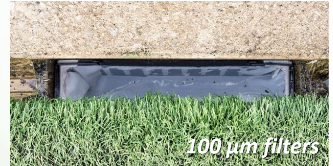
Filter system in the pitch water drainage
